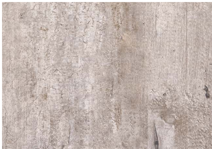
BN4 Cracked Concrete
